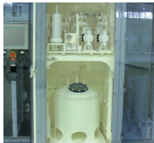
SIMONA® PVDF: Chemical mixing unit
